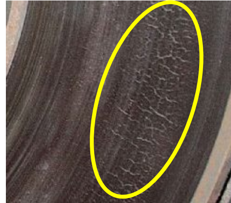
Visible cracking of the disc
