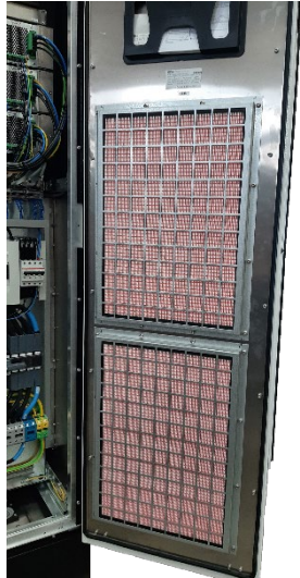
FIGURE 2: FILTER MATS IN THE RIGHT DOOR
