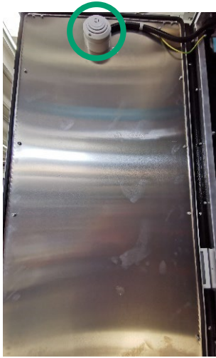
FIGURE 6: POSITION OF THE SMOKE DETECTOR
