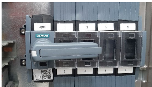
FIGURE 67: MAIN SWITCH "OFF"
